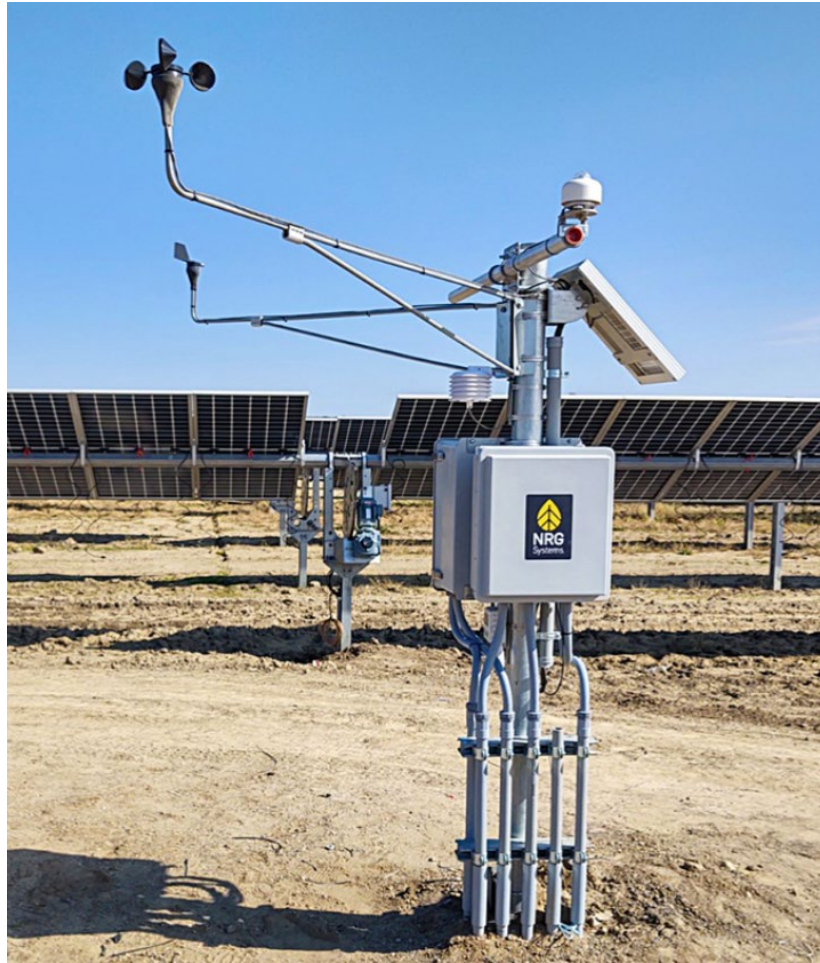
Figure 3.6.2-1 Typical Weather Station
